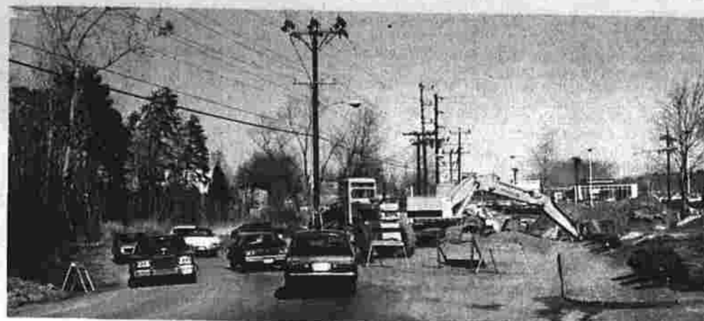
W. Middle Tpk. detour Motorists drive around a bypass on W. Middle Tpk. across from the entrance to the Parkade. The bypass was constructed to permit traffic flow while a new culvert is being built to allow water to flow under the road into Hilliard Pond. The old culvert was too small and occasionally caused flooding at the Parkade. (Herald photo by Pinto)
